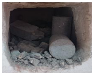
Figure 11. Explosive spalling occurs in cases of SCC and GFSCC mixes in 450 °C
