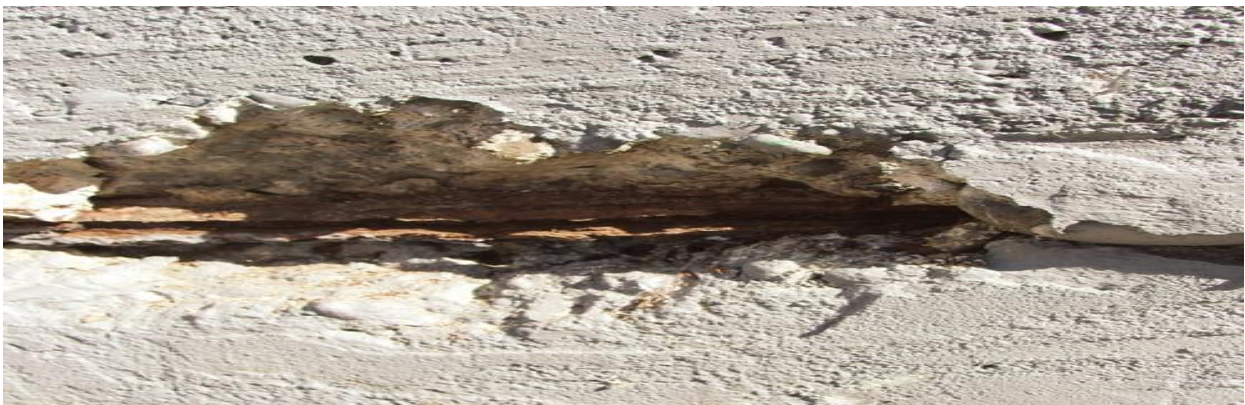
Fig 3 : Spalling due to rusting rebar.
