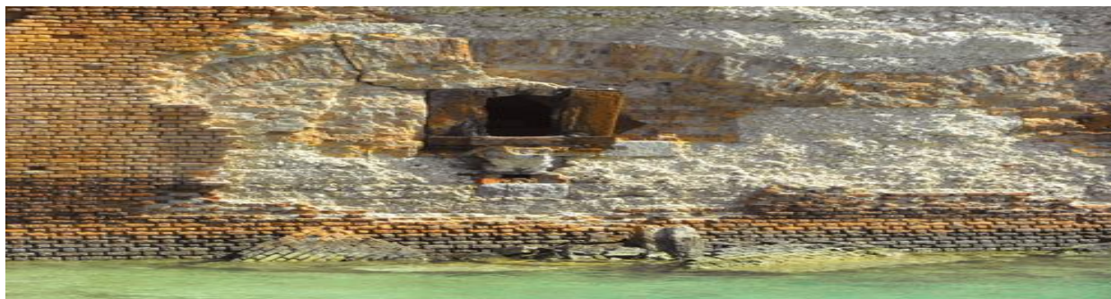
Fig 4 : A diagonal crack from expansion of rusting steel
